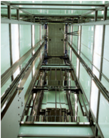
Lödige: lifts and escalators with state-of-the-art technology
