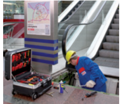
Maintenance on an escalator
