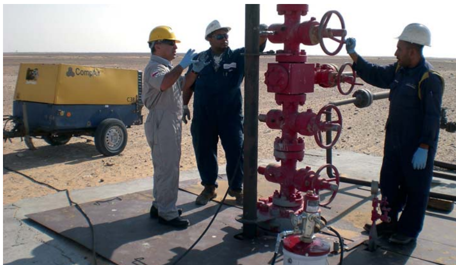
A „Christmas tree“ on an oilfield in Oman, which caps the well. Milispec supplies the special lubricants for the valves to make sure this is all completely secure.
