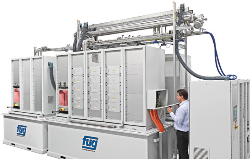
FuG power supply unit (600 kW, 40 kV) for a particle accelerator at BESSY in Berlin. Windows and mirrors for the visual inspection of the oil condition and switch position of certain safety-relevant parts.
