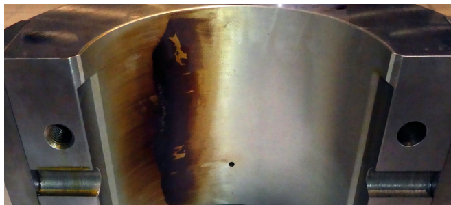
View into a pinion bearing: Before ...
